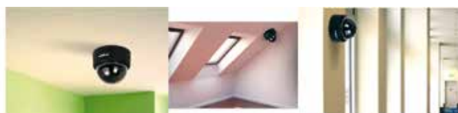
Camera installed on the ceiling
